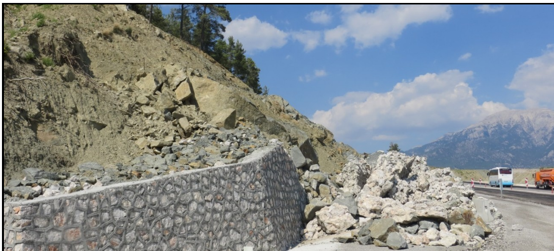
Photograph 3. The Landslide Forming at the 10.th Kilometer of Kemer-Antalya Highway from Time to Time Hinders the Highway Traffic.
