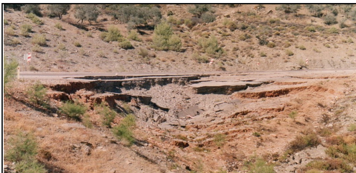
Photograph 2. Damaged Highway of the Landsliding Region in Kemer-Antalya Highway's 5.th Kilometer
